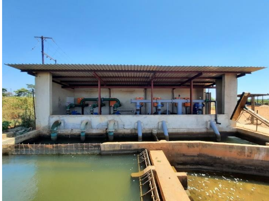
Figure 18. Three pumps for the SDI system (light blue-grey, on right side picture)
