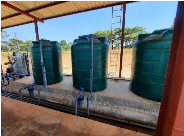
Figure 21. Fertigation tanks SDI system KASCOL
