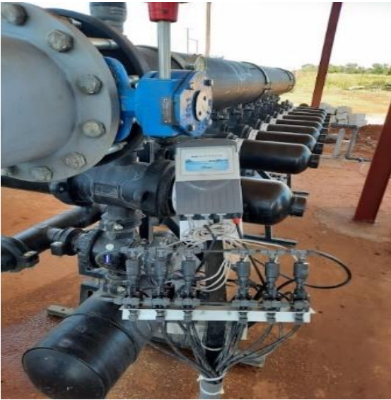
Figure 19. Main screen filtration system SDI at KASCOL
