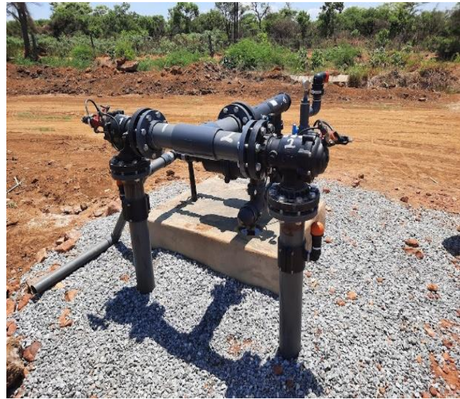
Figure 20. Secondary filtration station
